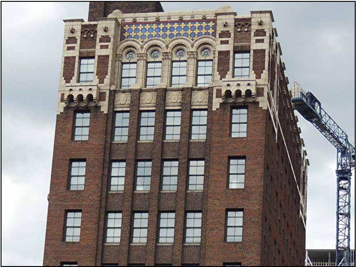
Note the darker brick, which appears to be staining, in the center area of the building.
