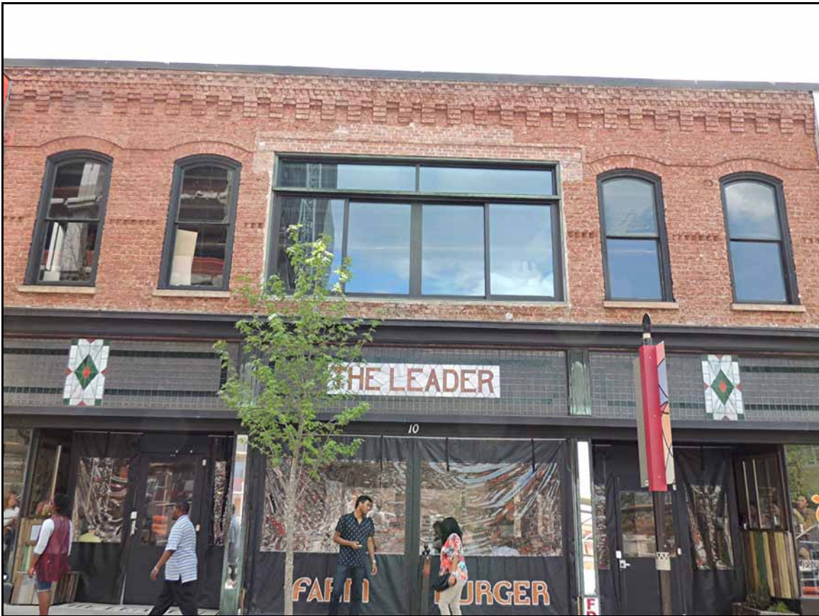
This building front has some nice brick work that has been pressure washed. Note the repair work done above the large window.
