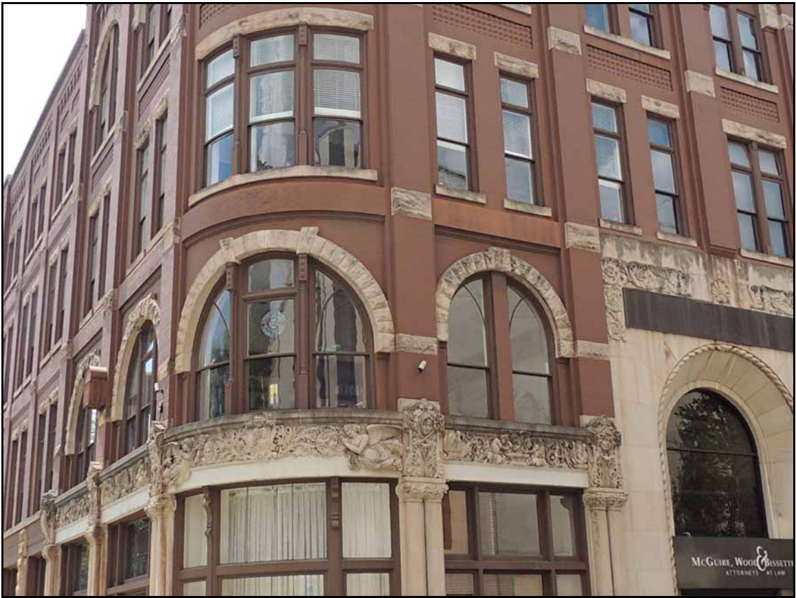
Note how the staining on the stone starts at the top and works its way down.
