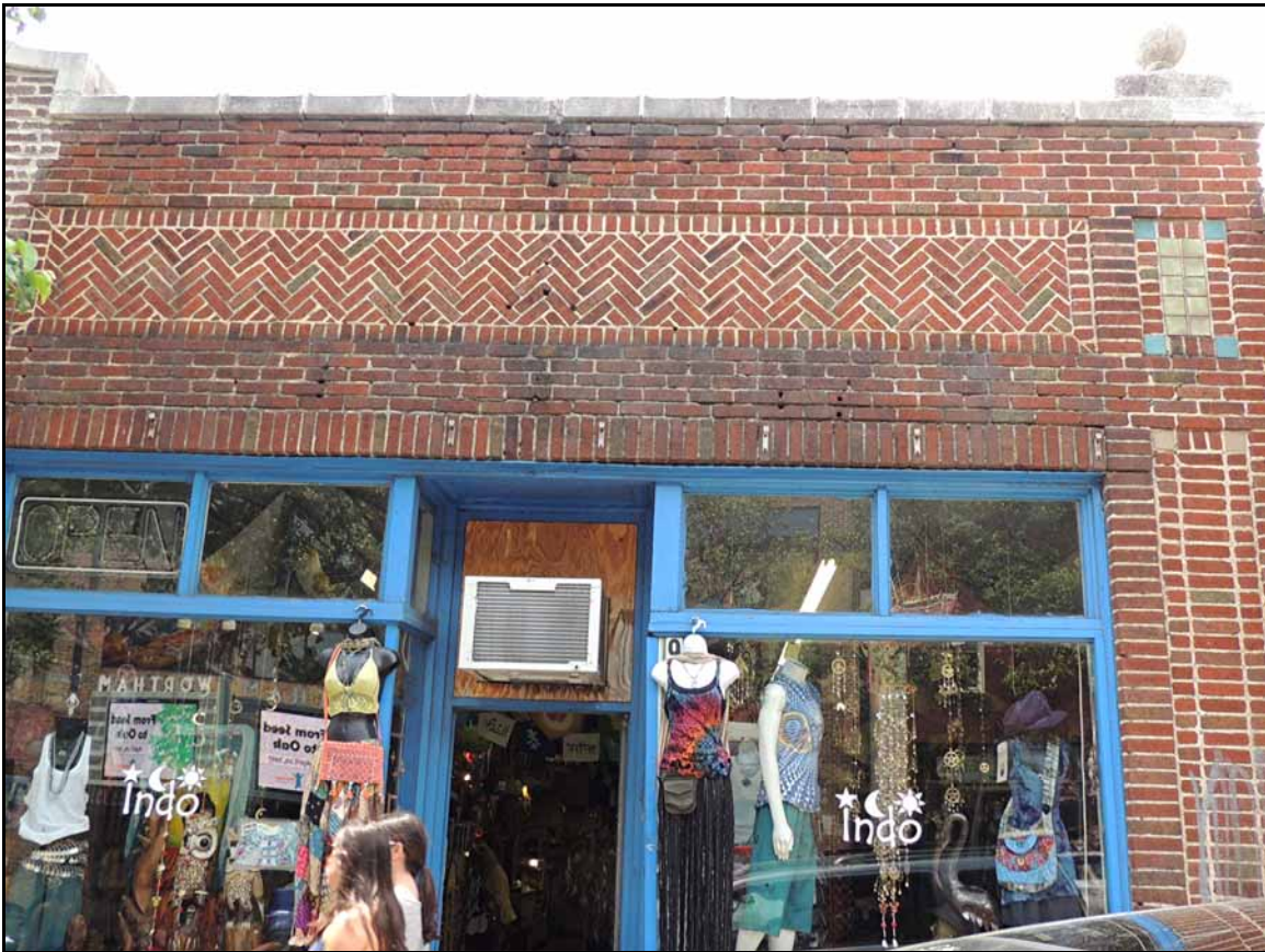
Another interesting brick pattern and the mortar between the bricks appears to be consistent on this building front.
