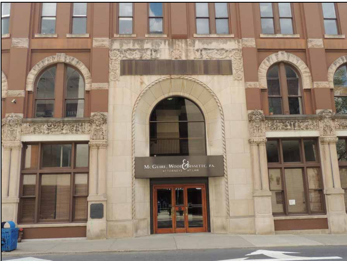
The 11 stone sections for the arch above the door are set equally. There is no noticeable key stone at the center of the arch. The carvings in the stone are beautiful. Note the mild staining at the top of the stone and the heavier staining on the carvings.
