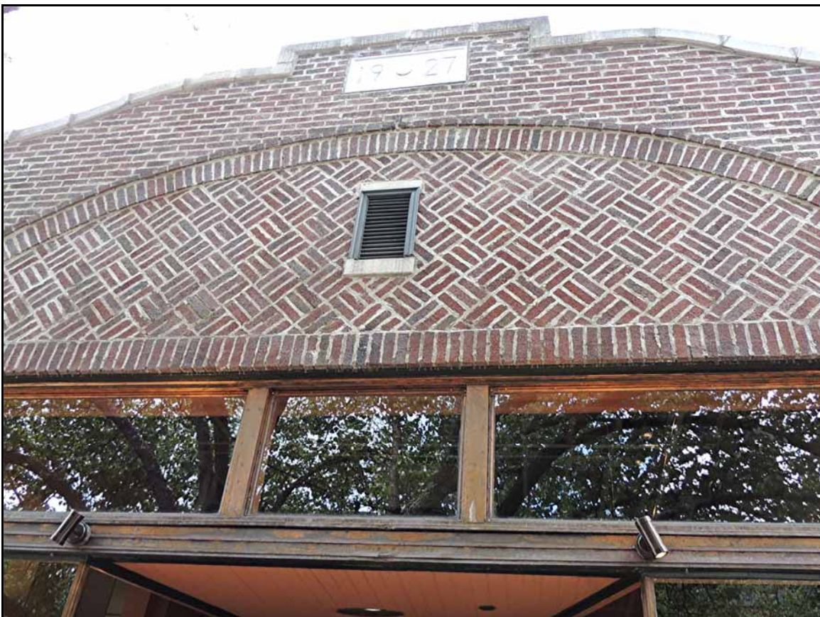
Note the spacing between the bricks on this building front and the increased amounts of mortar used to set them.
