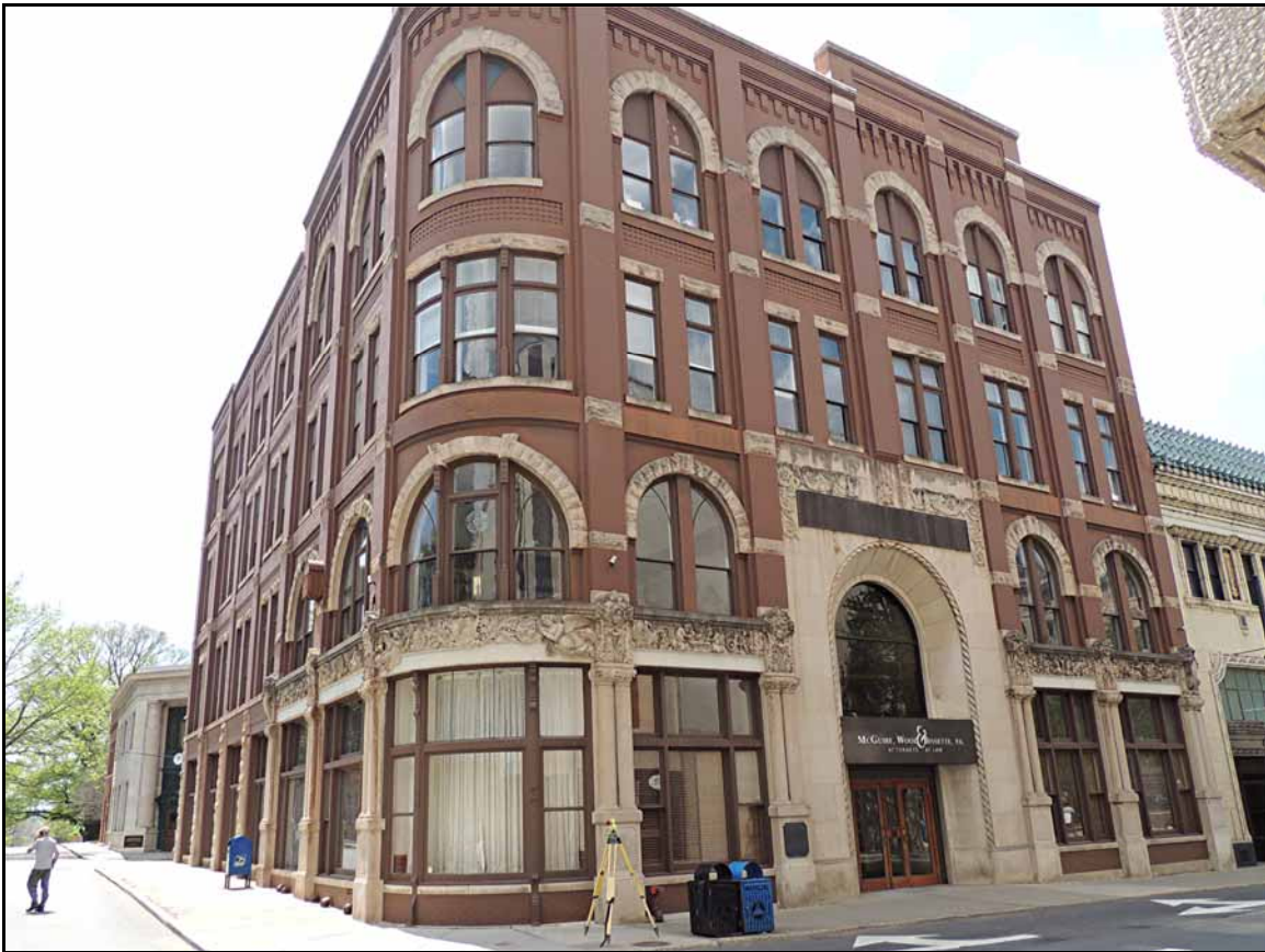
Note the brick work and how the stone on the tops of the windows is set.
