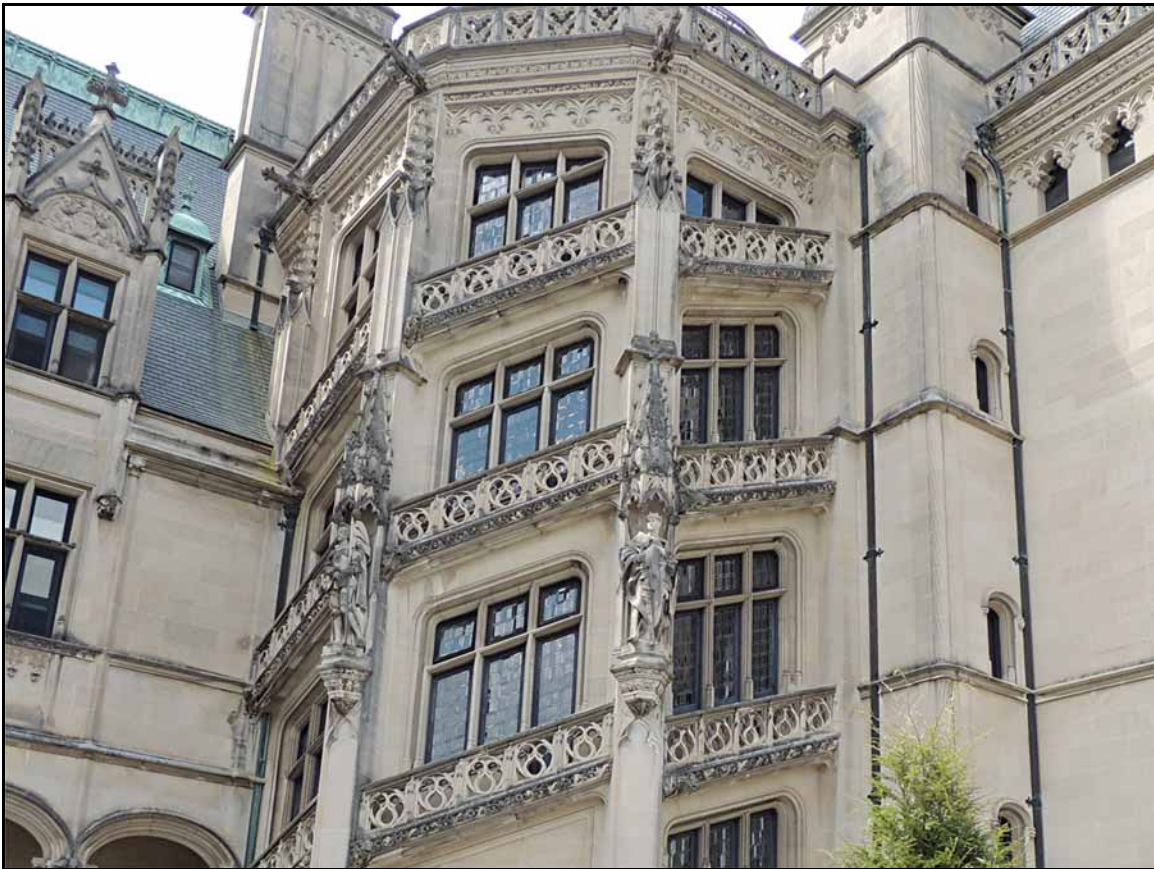
A close up of the stone carvings and statues show how much craftsmanship went into their creation. Note the color of the metal rain downspouts. The mold and grime is on the undersides of the stone carvings.
