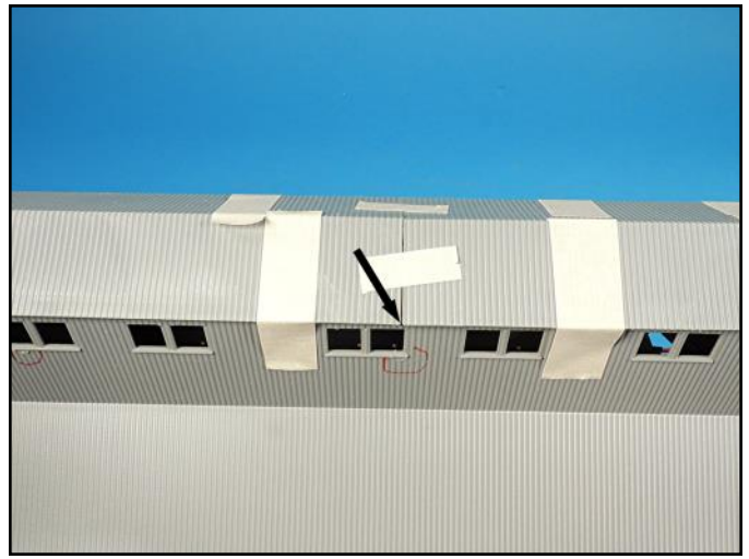
The roof comes in two sections and there is a gap which will need to be fixed.
